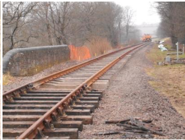
The last panel at Monteswood Lane Bridge connected to last year's replacement.
