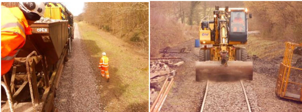
Matt Crawford walking alongside the moving ballast wagons immediately followed by the plough driven by L&W expert driver, Darren. Photos from 2018 relay.
