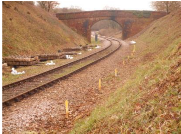
Part 2 ready to start at Caseford Bridge adding 13 panels to last year's snow covered relay.
