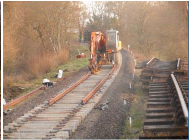
Progress at the end of the following Tuesday with Sloop bridge in the distance.
