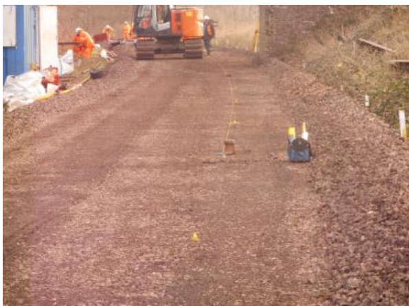
Marking the line slightly further from the bridge wall blending back onto the original course.
