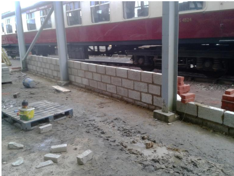
The interior blockwork of the dwarf wall on the western side of the maintenance road (Bruce Healey).
