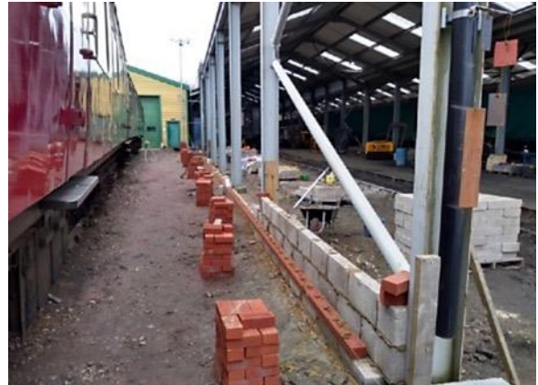
The photo shows the beginnings of the dwarf wall on the western side of the maintenance road.
