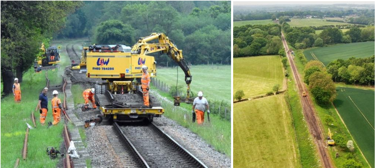
Track removal viewed from the signal post and from John Harwood's drone.
