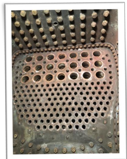
Right: Firebox tubeplate, showing the tubes and flues released prior to removal.
