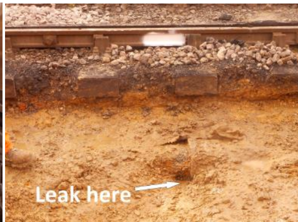
Leaking pipe found and marked.
