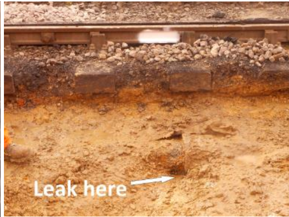
Leaking pipe found and marked.
