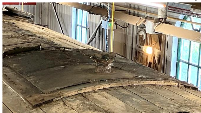
Water tank and (top left of picture) a monsoon vent, still in situ after removing the roof covering and the wooden tank cover. April 2024
