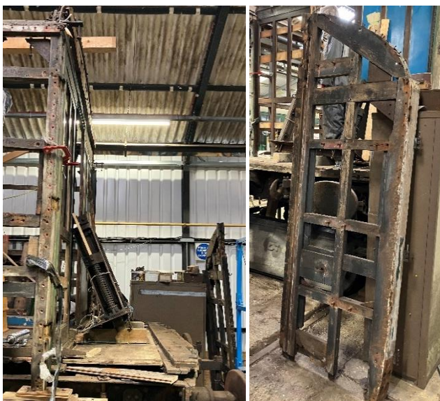
South vestibule after taking down the gangway plungers and end frames; SE end frame. July 2024
