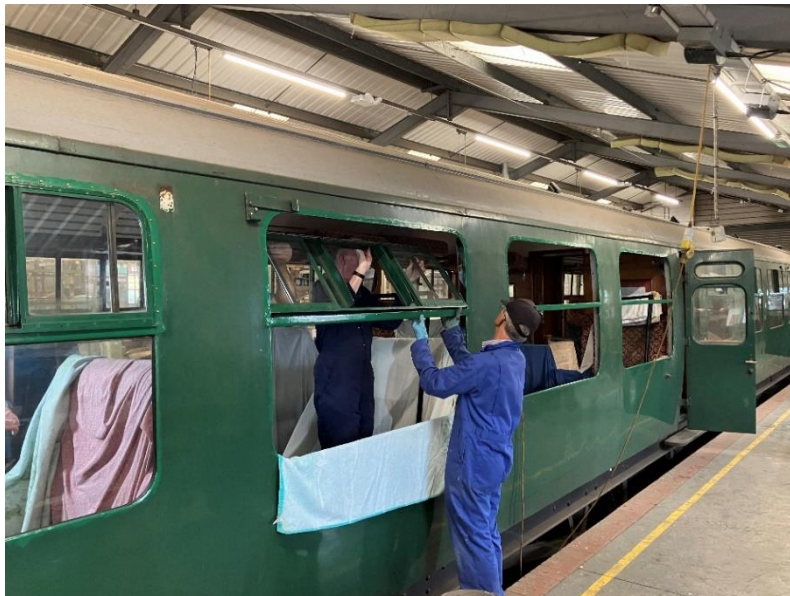
The second of the four top light assemblies being reinstalled in 1482's northern saloon. July 2024
