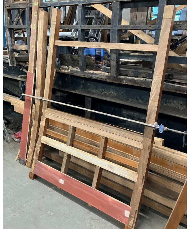
The replacement frame section for the west side; shown is its inner face. Aug 2024
