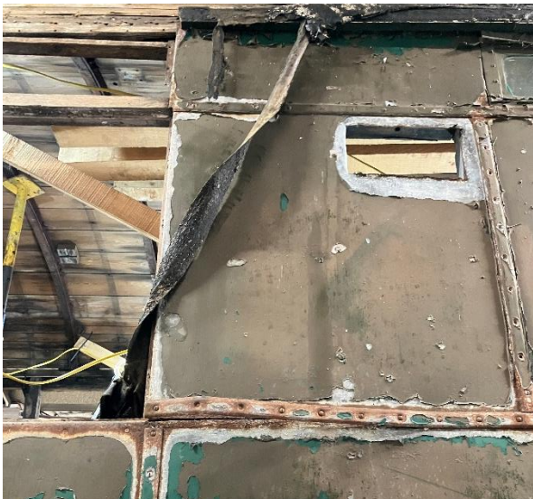
Steel panelling detail showing the joint cover strips and returns into the window opening. March 2024
