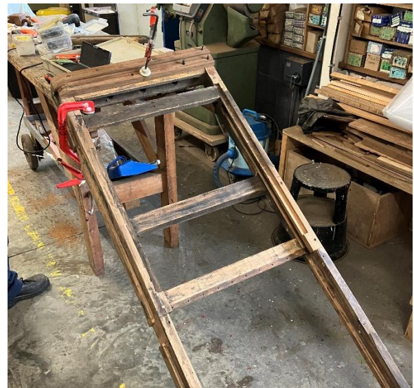
One of the doors from the west side double-door pair under repair; a new bottom moulding has just been added. Sep 2024
