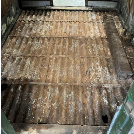
Floor of a compartment after removal of the decolite layer. The floor is set in a 1 ½" rebate in the frame timbers on all four sides. 4 Mar 2026
